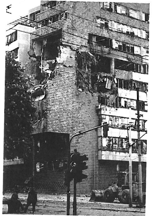
▲ General headquarters of the Yugoslav army in Belgrade, damaged during NATO bombing
